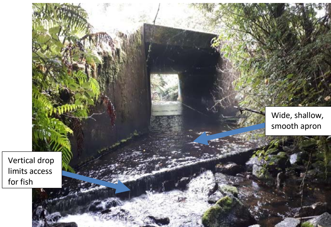
Figure B-17: Fish movements will be impeded by the fall at the downstream end of the apron and shallow water on the apron. Photo credit: Sam Ammon.
