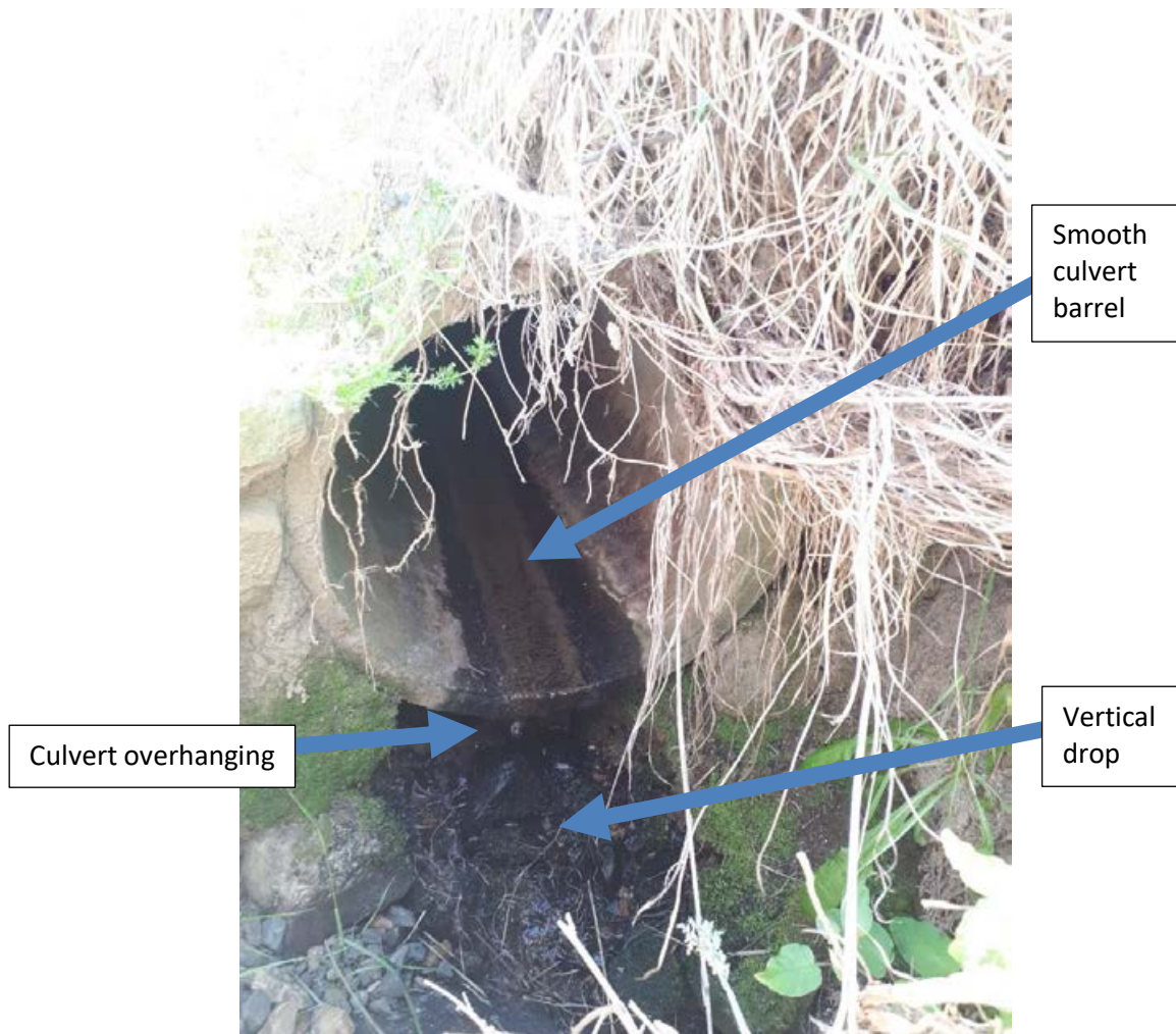
Figure B-15: Fish passage will be impeded by the fall height and undercut at the culvert outlet. The smooth culvert barrel will also lead to higher water velocities and limit fish movements under higher flows. Photo credit: Megan Brown.
