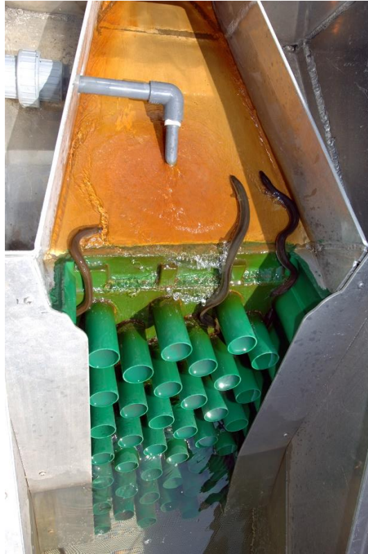
Figure 7-11: Milieu Inc. Eel ladder (for eels 150–750 mm) installed at the Moses-Saunders Dam. Photo credit: NY Power Authority.
