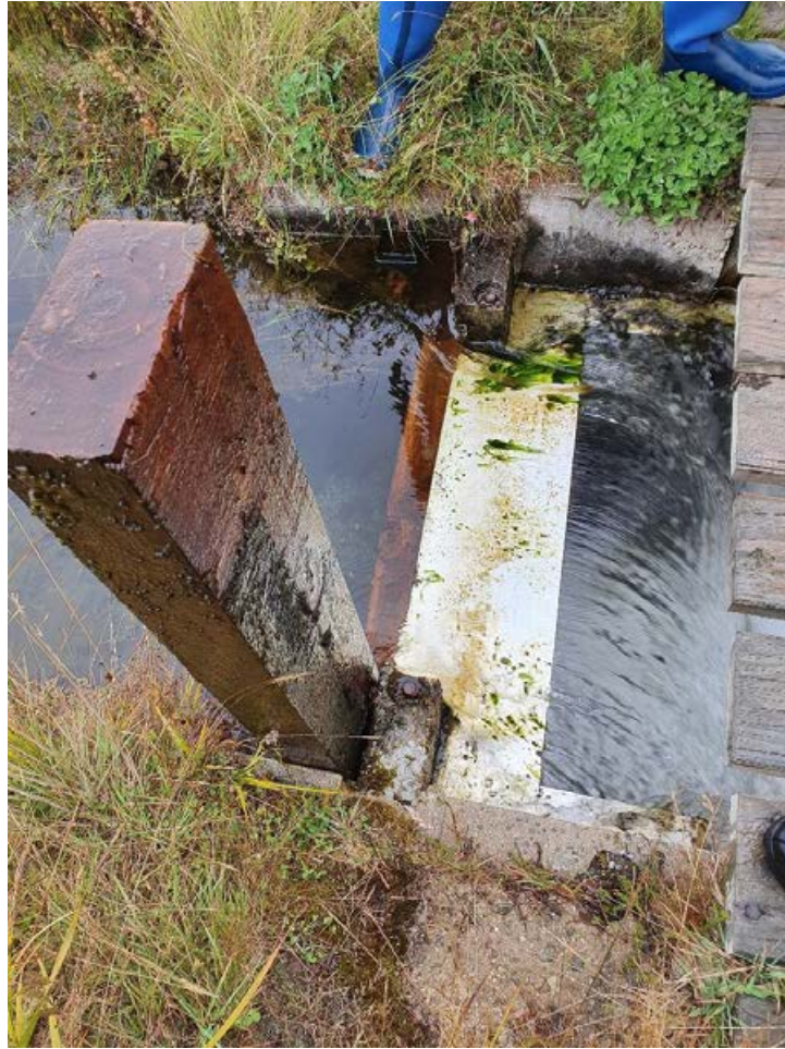
Figure 6-18: Wooden slots on the Fraser Spring exclusion barrier that can be manually removed to flush sediment and lower water levels (photo showing one removed). Photo credit: Sjaan Bowie.
