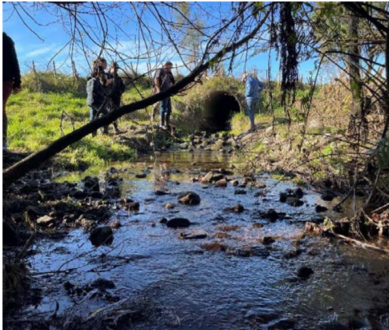
Figure 5-15: An example of a grouted concrete rock ramp below a culvert in the Manawatu-Wanganui region. Top, as built in 2014. Bottom, a decade later in 2024. Concrete is used to prevent water seepage between rocks and is shaped to provide a low flow channel and resting pools to facilitate upstream passage. Photo credit: Cindy Baker.
