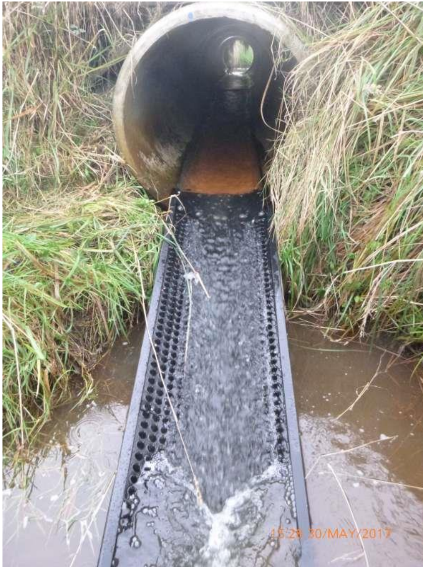
Figure 5-22: Example of an artificial fish ramp installed at a perched culvert in Southland containing the Miradrain™ substrate. Note that a shallow wetted margin is maintained on both sides of the ramp. Photo credit: James Dare.
