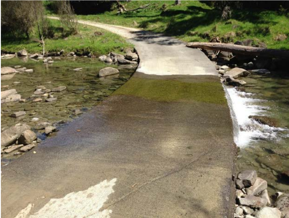
Figure 4-21: Raised roadway ford crossing. The vertical drop on the downstream side will block fish movements. Shallow water depth and elevated water velocities across the ford pavement can also impede movements.
