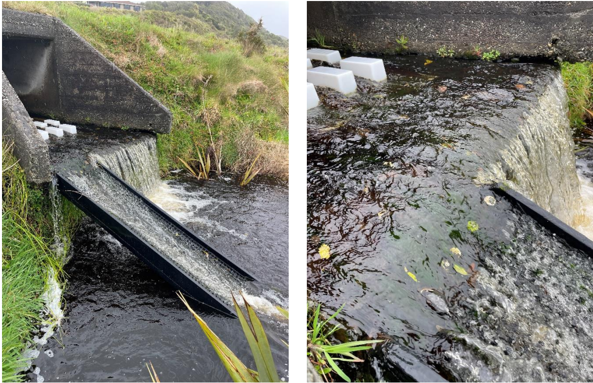
Figure 5-24: Artificial substrate ramp installed at a perched culvert on the West Coast. There are multiple ways this installation could be improved. Left: The entrance to the ramp extends past the upstream limit of migration and the ramp is too steep (~35°). The end of the culvert apron is also left unbaffled, which creates a high velocity impediment for any fish able to surmount the ramp. Right: Close-up of the ramp crest showing a high velocity barrier created by the smooth flexible crest used for ramp attachment and the lack of baffling at the crest. Note: this substrate is not Miradrain™ (see Figure 5-20 & Figure 5-21). Photos: Cindy Baker.
