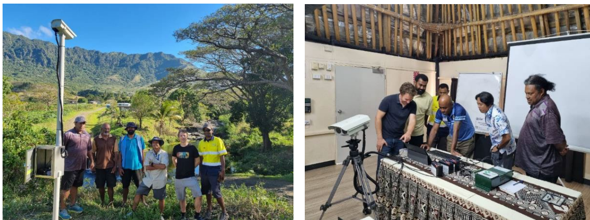
Stereoscopic camera station installation - Narara Village.
