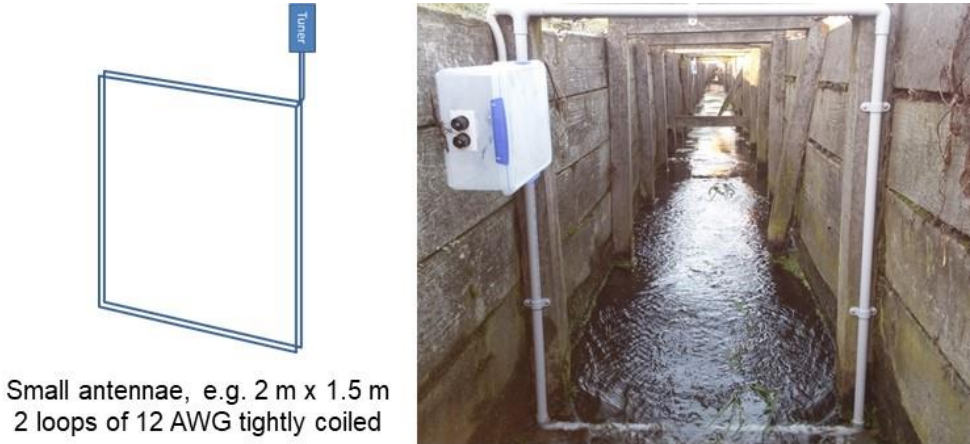
Figure 6-17: Double coil PIT antenna design. Antenna wire is housed within conduit piping for mechanical protection. Abbreviations: AWG, American wire gauge.
