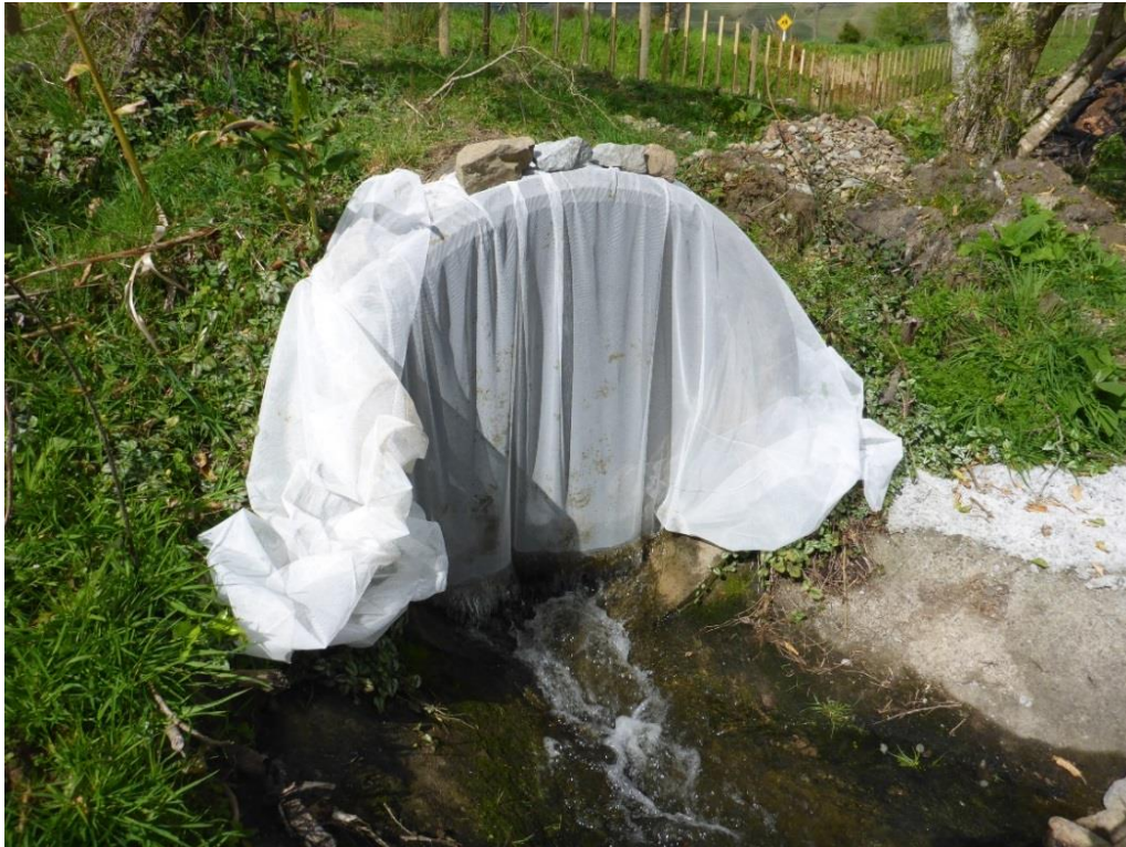
Figure B-2: Barrier net set upstream of the baffle at the culvert outlet.
