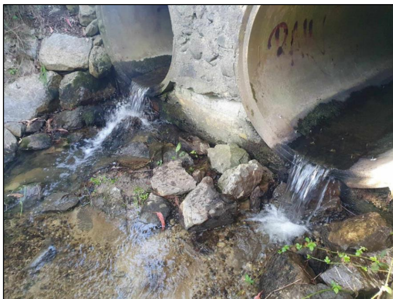
Figure A-3: Perched culverts at Williams Creek pre-remediation. Photo: Tim Olley.
