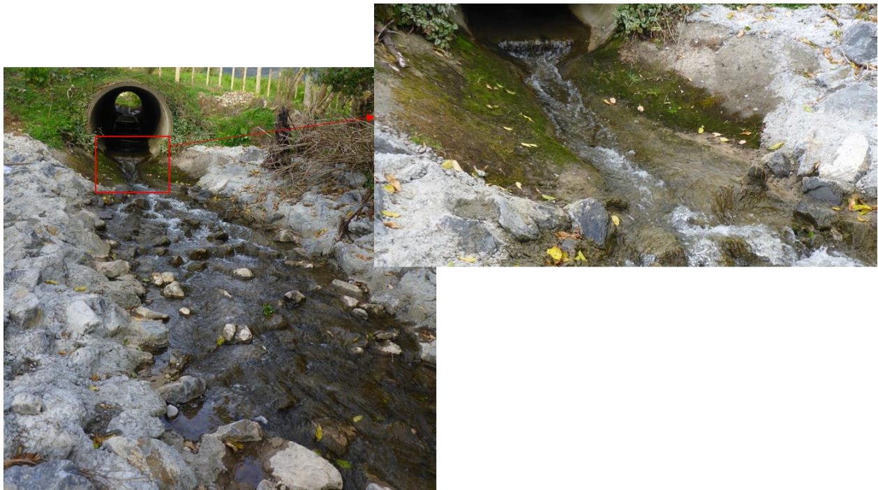
Figure B-1: Remediated culvert on Kara Stream, Upper Kingston Road. Inset shows the unmodified culvert apron.
