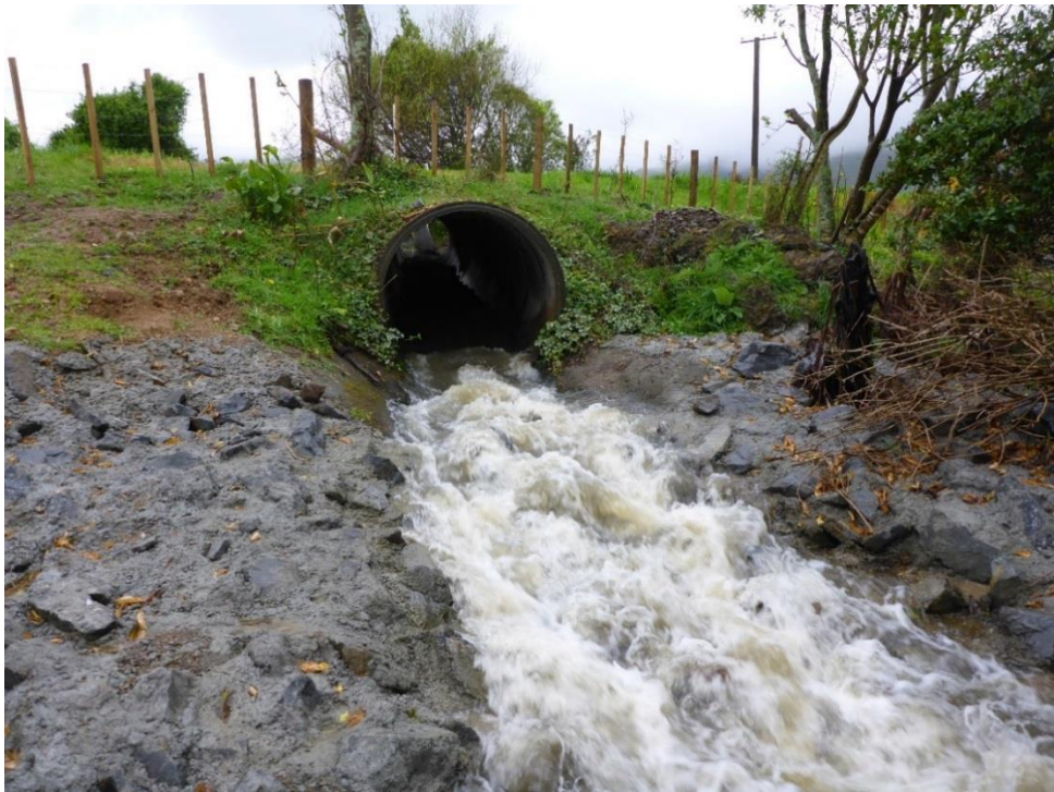
Figure B-2: Flow through the culvert and over the rock-ramp at the conclusion of Trial 3.
