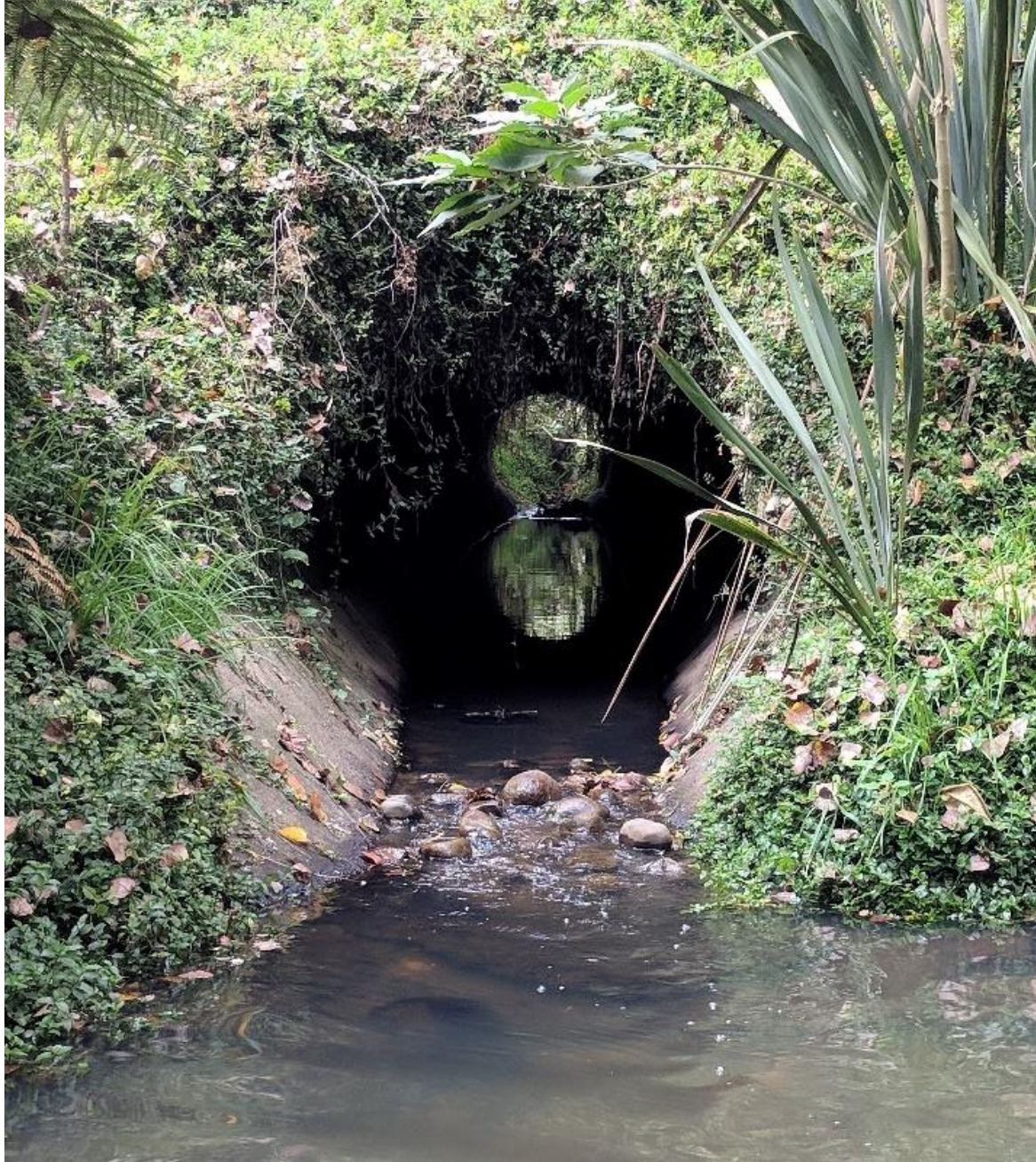
Figure C-2: After remediation of the culvert apron and installation of baffles in Waterford Road culvert in Mangakotukutuku Stream, 2019. View from downstream looking upstream through the culvert.
