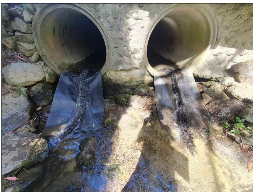
Figure A-4: Post-remediation at the Williams Creek culverts, showing two flexible rubber ramps with mussel spat rope. Photo: Tim Olley.
