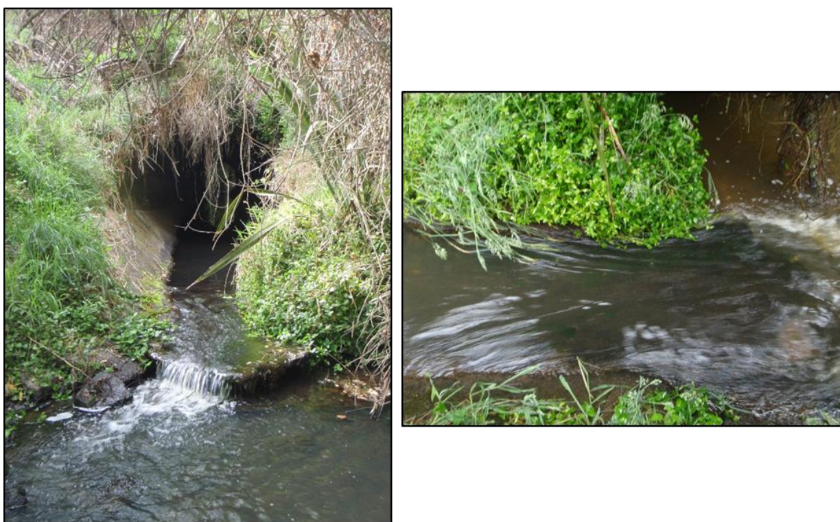
Figure C-1: The outlet of the Waterford Road culvert. Perching of the apron at low flows (left) and high water velocities across the apron (right) create a barrier to upstream passage of fish.
