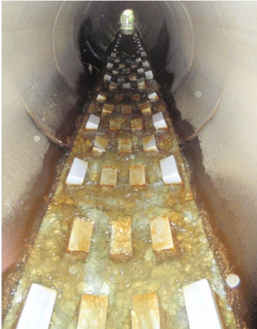
Figure D-2: The culvert barrel following installation of the spoiler baffle sheets.
