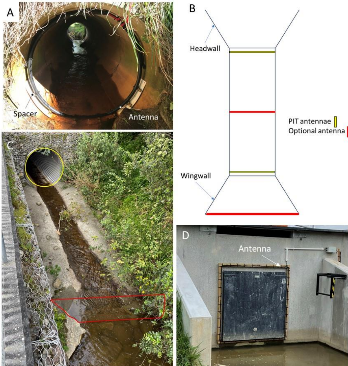
Figure 6-14: Passive Integrated Transponder (PIT) antenna setup at a culvert. A, PIT antenna installed inside a pipe culvert. Note the spacer necessary to avoid the electromagnetic field being dampened by the steel reinforcing inside the culvert. Although the antenna wires are raised from the culvert base, the read range of the antenna extends to the culvert floor. B, Plan view of a typical culvert arrangement showing the conceptual placement of PIT antenna to monitor fish movements over the apron and through the culvert barrel. C, Mark-up of a pipe culvert and rock ramp showing the placement of an antenna at the base of the rock ramp and inside the culvert outlet. With an antenna at the culvert inlet, this system will determine passage efficiency across the rock ramp separately from passage efficiency through the culvert barrel. D, antenna placed around the outside of a metal gate at a pump station culvert outlet.
