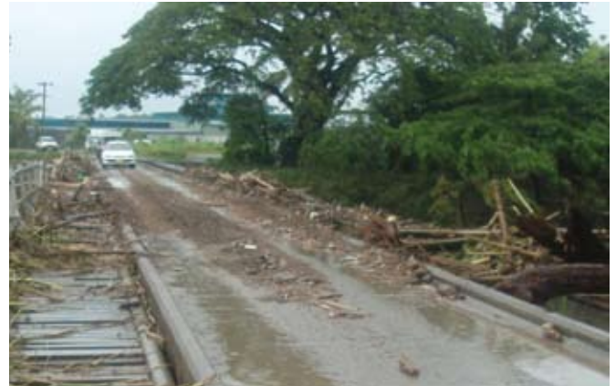
A badly damaged bridge in Nadi, Fiji
