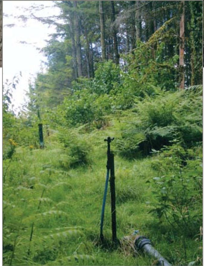
Spray irrigation of treated sewage effluent into Whakarewarewa Forest in Rotorua. The groundwater ecosystem removes some of the contaminants (including organic carbon) entering the shallow groundwater here, as well as at most other sites where effluent is variously discharged to land.
