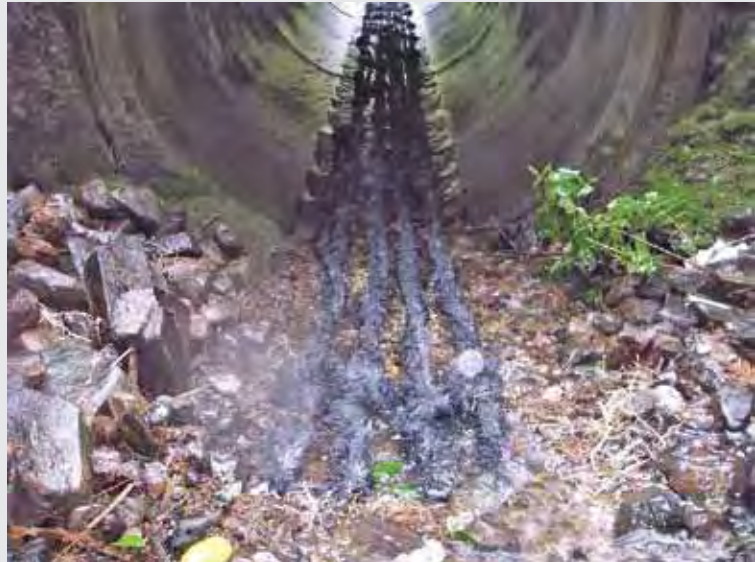
Textured ropes installed in a stream culvert to aid fish passage. Photo: Bruno David
