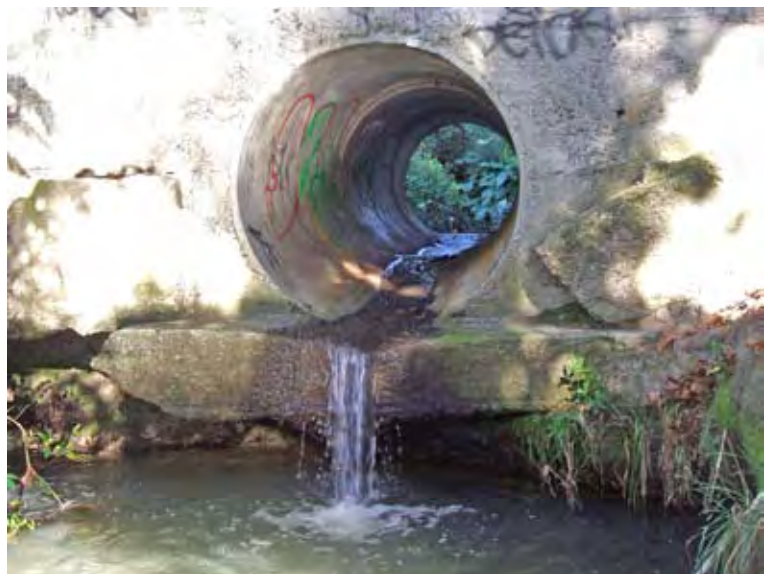
Example of potential barriers to fish passage: perched culvert.
