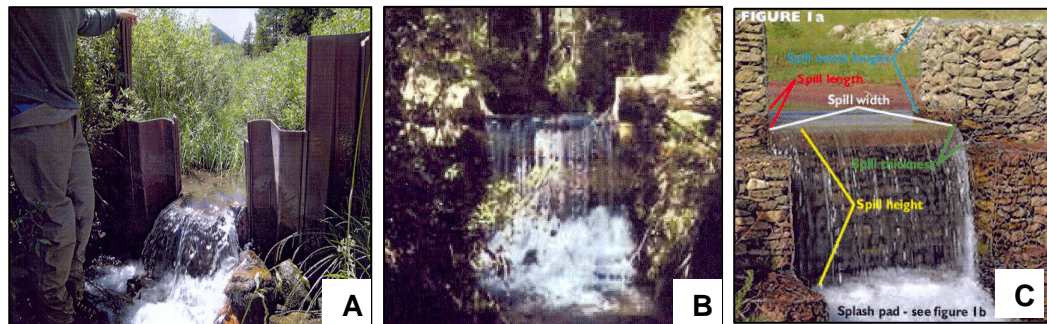
Figure 10: Different ways of constructing weirs at low head sites; (A) interlocked metal sheets (i.e., coffer dam) rammed vertically into the substrate, (B) log or wooden planks laid across the stream channel, (C) rock-filled gabion bags with the spill height and splash pad designed to prevent upstream passage of salmonids. (Photos are from www.wildfish.montana.edu/projects/barrier/browse.asp ).
