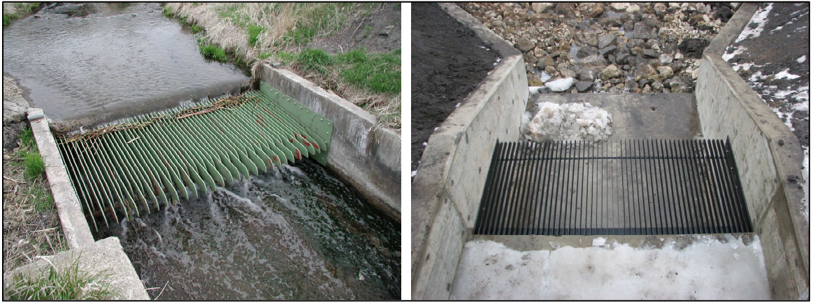
Figure 22: Examples of low-head protruding bar screens designed to prevent fish from jumping the crest of the weir. Such screens also act as trash barriers (cleared during flood flows) and provide a length of de-watered channel which is a further deterrent to fish upstream movement (photos courtesy of Nicole Hansel-Welch, Minnesota Department of Natural Resources).
