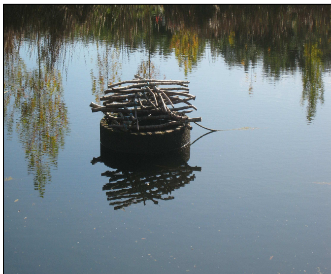
Figure 13: A well or stand-pipe provides the outlet to a small pond created by a weir and maintains a constant water level in it. The well entrance can be screened to prevent waterfowl or debris from falling into the well. A horizontal culvert at the base of the well ducts water under the pond and away to the nearest water course.
