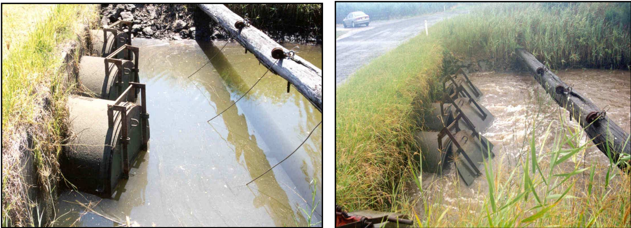
Plates 1 & 2: Floodgates during non-flood and flood times respectively
