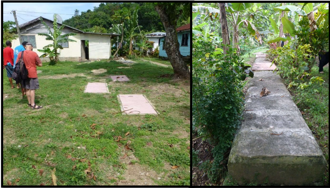
Figure 4-2: Land application trenches sampled in Namaqumaqua showing inspection hatches. The House 1 LAS (left) was set into the existing sandy soils on the seaward side of the village, and the House 2 LAS (right) was set in a raised bed above the clay soils and shallow water table on the landward side of the village
