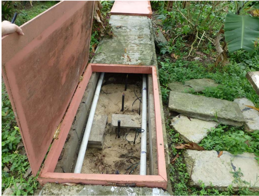
Figure 4-3: Raised bed LAS sampling point for House 2 clay soil site. Wastewater dosing distribution pipes (white) pushed to side of trench. Fullstop™ samplers and tubes enabled samples to be drawn from the bottom of the sand filter.
