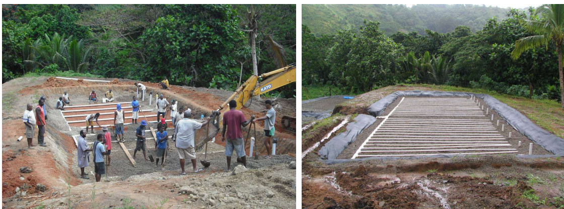
Figure 5-5: Votua Vertical flow wetland during construction. The photos show basal drainage pipes being covered in gravel (left) and surface dosing pipes (right).
