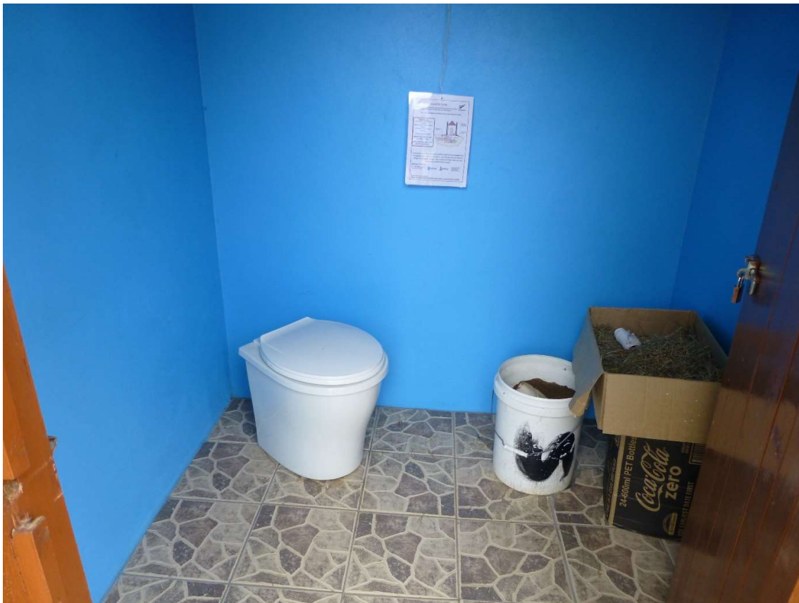
Figure 2-6: ecoVIP2 pit latrine interior at Bavu. Note soil and mulch material available to add into the toilet after each use.
