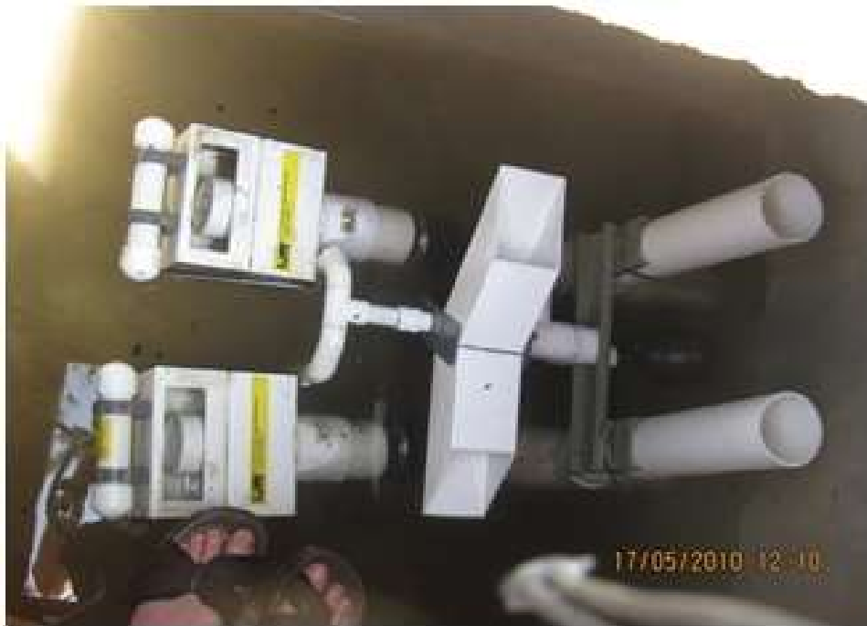
Figure 5-4: Alternating flouts in VFCW dosing chamber.
