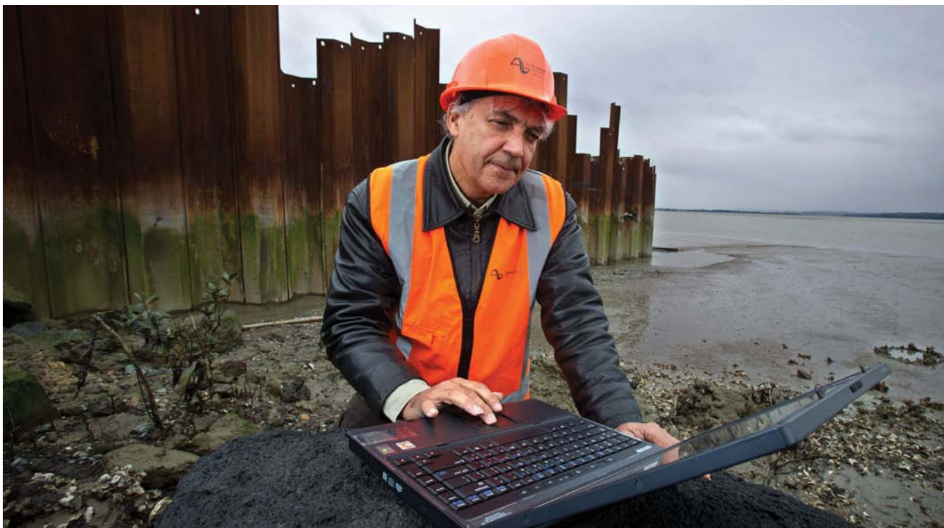
NZTA Principal Environmental Specialist, David Greig, monitors sediment transport beside the northwestern motorway reconstruction, in west Auckland. "We need to keep check on the sediment load into a sensitive environment." (Geoff Osborne)
