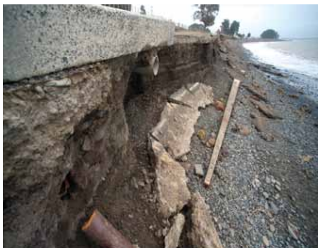
At Clifton, near Havelock North, waves have damaged stormwater infrastructure and undermined the road that services the Clifton campground. [Dave Hansford]
