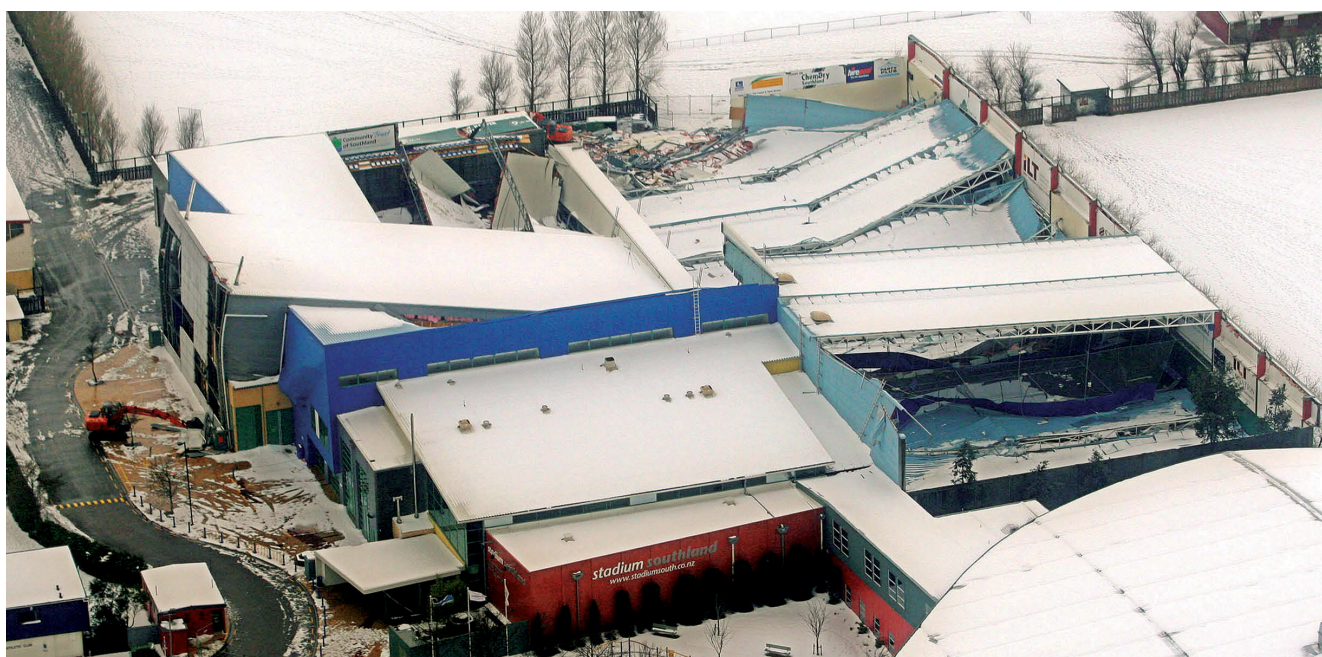
The Southland Stadium lies flattened after the September, 2010, snow storm. Department of Building and Housing subsequently identified faulty remedial work to fix sagging roof trusses, along with welding that was either substandard or missing altogether. Police found no evidence of criminal liability. Invercargill City Council now faces a $27 million lawsuit from the building’s owners. ( Southland Times )
