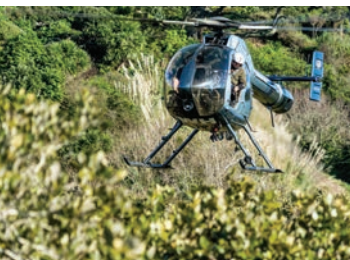
Another payload of pipes and poles is deployed among the mangroves in the Athenree estuary. (Lana Young)
